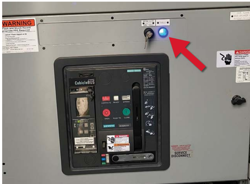
Leaving the maintenance bypass switch enabled reduces power system reliability.
