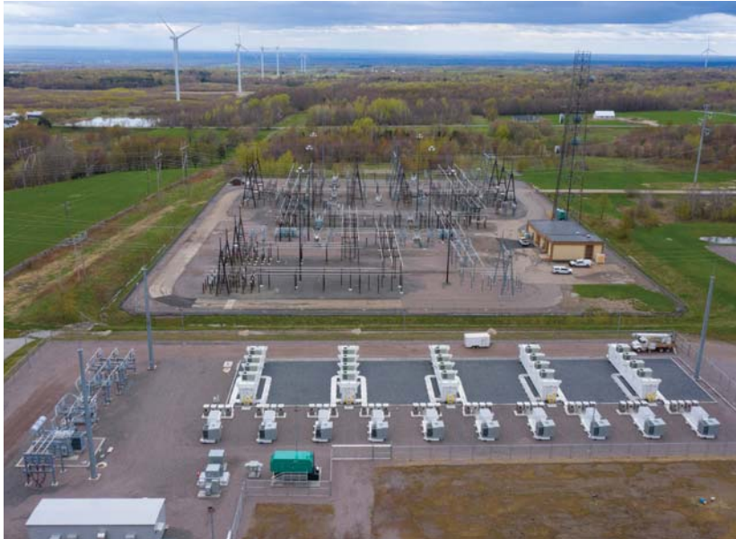
Drone view of the Northern New York battery storage project, with construction completed. The Willis substation is adjacent to the facility.
