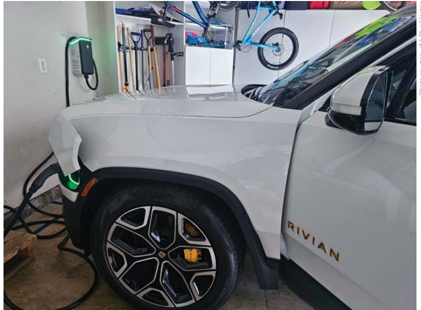
Photo courtesy of A Plus Electric
