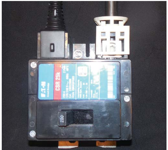
Photo 1. Protective barriers are permitted to be installed on the supply-side terminals of a circuit breaker used as a service disconnect.
