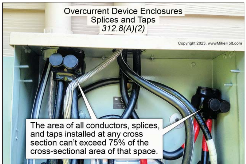
Fig. 2. Splices and taps can be placed in the wiring space within panelboard cabinets as long as the space they take up doesn't exceed cross-sectional area limitations.
