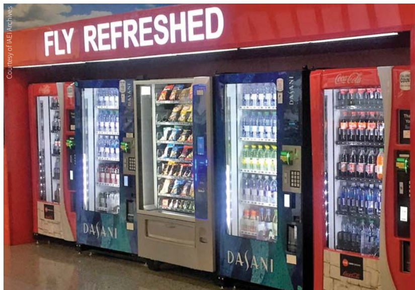
Photo 1. Section 210.8 of the NEC specifies ground-fault circuit interrupters (GFCIs) must be installed in a readily accessible location, such as in the case of vending machines.
