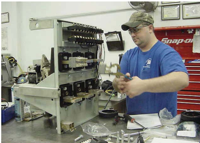
Photo 1. A technician working on a low-voltage power circuit breaker.
