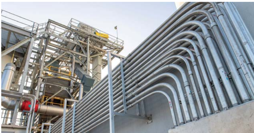
The Interstates team collaborated closely with the other project partners to preplan model conduit racks on the Ardent Mills Port Redwing Flour Mill in Gibsonton, Fla.. The model allowed the team to move some work into the early stages of the project, increase the installation rates, avoid clashes with other installations, and review the routing with the owner.
