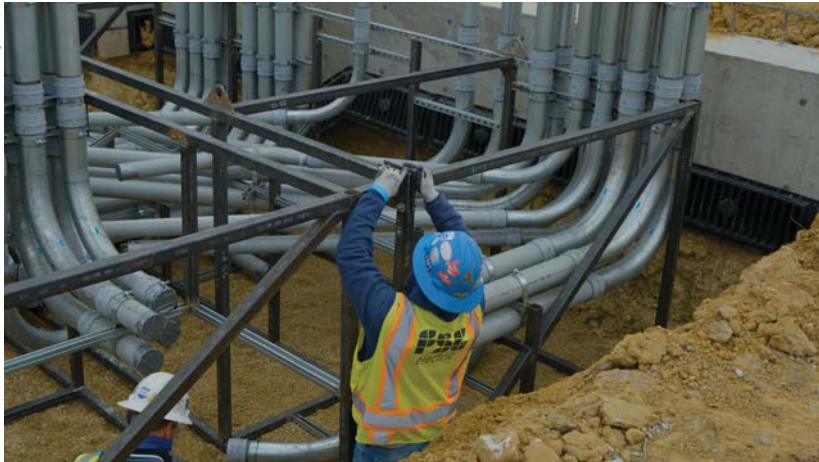
In Denton, Texas, a prefabricated underground utility service rack was delivered to a hospital expansion project site on the day it was scheduled to be installed by FSG.
