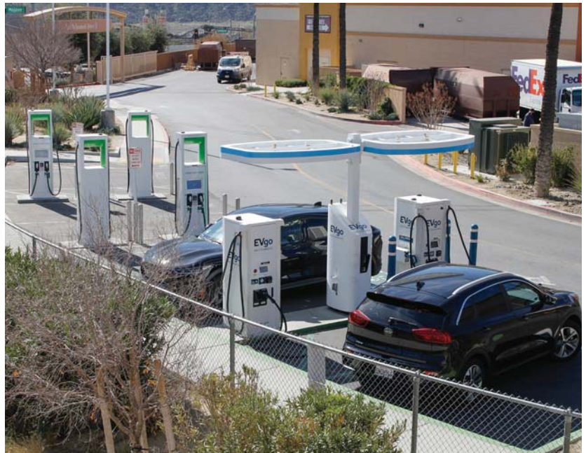
Photo 1. One of the major considerations for building out electric vehicle charging infrastructure is determining what level chargers will be needed. This decision will affect the design and cost.
