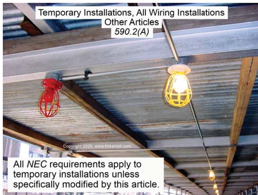
Fig. 1. If you have a temporary installation, you don't just apply the requirements of Art. 590 and consider the installation Code-compliant. Instead, you apply the relevant requirements of Chapters 1 through 4, and check Art. 590 for modifications of those.
