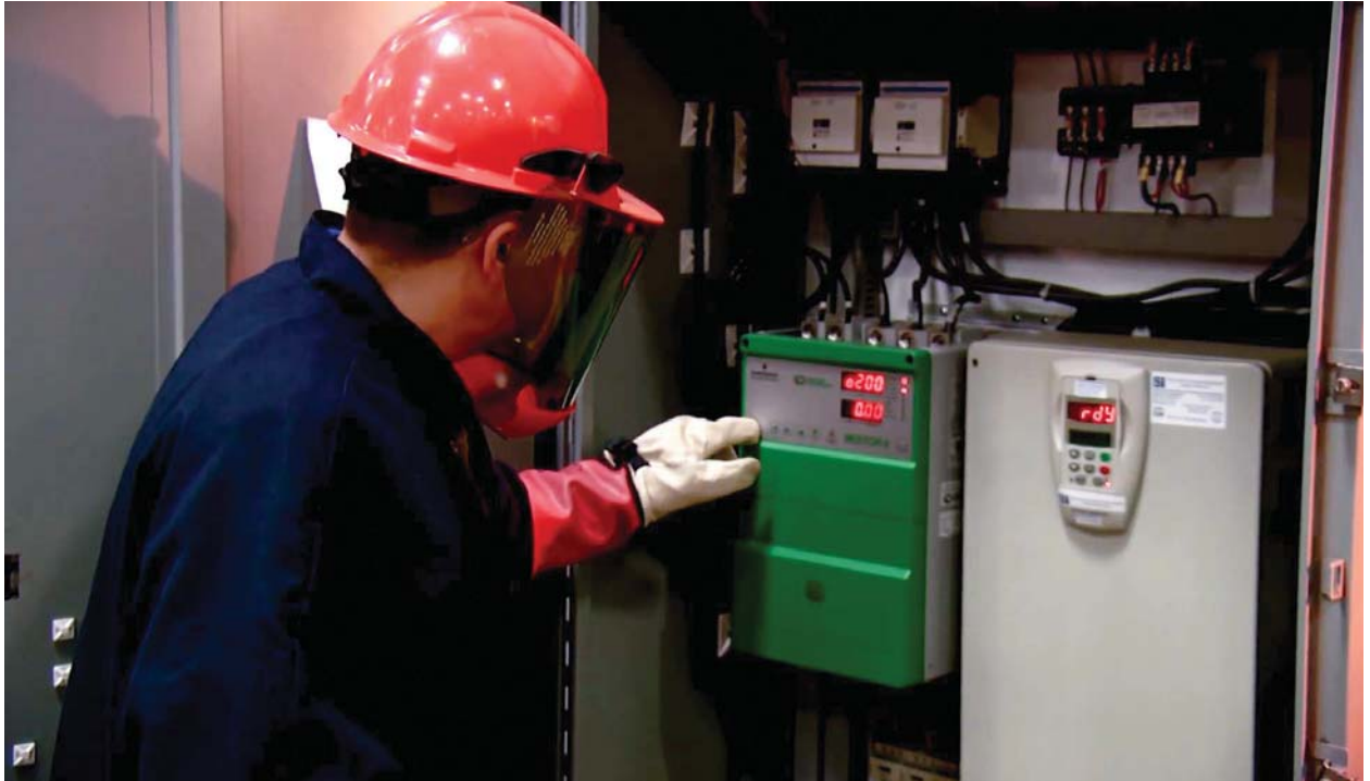
Understanding safe working procedures empower electrical contractors to tell a customer “no” when safe conditions cannot be met.
