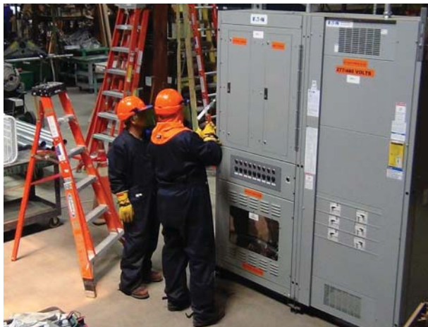
Sturgeon Electric’s energized work training puts trainees in front of de-energized equipment.
