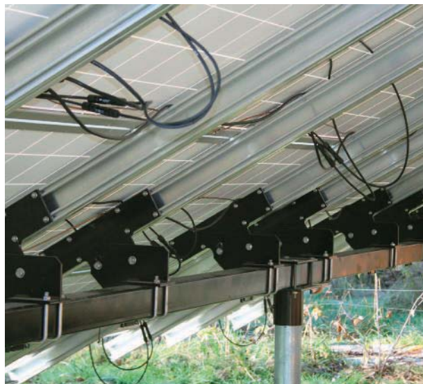
Photo 2. Unsupported conductors can result in damage to the PV system and put anyone in contact with the array at risk of electrical shock. Not only are the conductors of this array not supported properly, but they also are considered readily accessible and would require proper protection.
