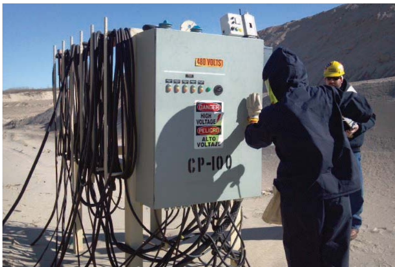
Team members test/troubleshoot a portable PLC/power distribution unit for portable mining equipment.
