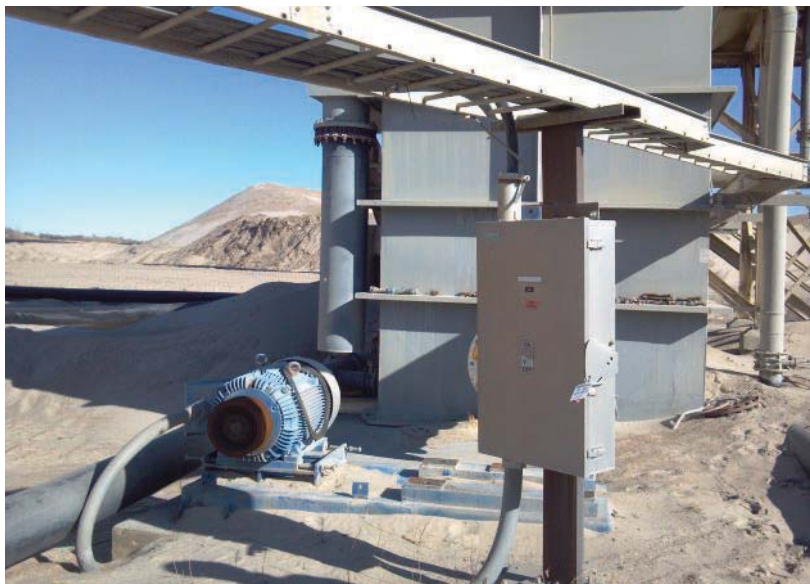
The slurry tank shown in the background is where sand and water are combined to create the pumpable slurry mixture that is sent from the mine site down to the wet plant for processing.
