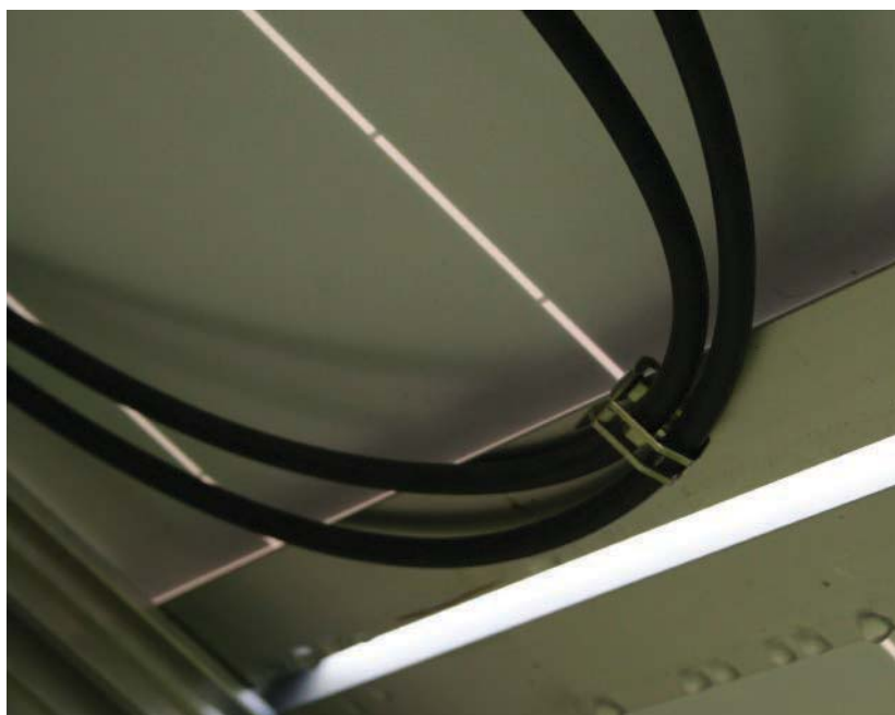
Photo 1. Conductors that are properly supported to the module frames are less likely to cause long-term problems. Various products are now available that are designed to clip to the module frame and hold PV conductors in place.
